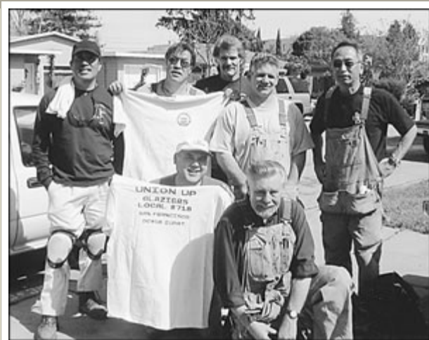
Glaziers 718 volunteers replace windows at the home of Geri Warren, wife of the late Stan Warren. L-R: Richard Lucha, Leland Wong, Larry Stavosky, Nick Barulich, Doug Yamamoto. Kneeling: Dan Angel, Steve Zuniga
